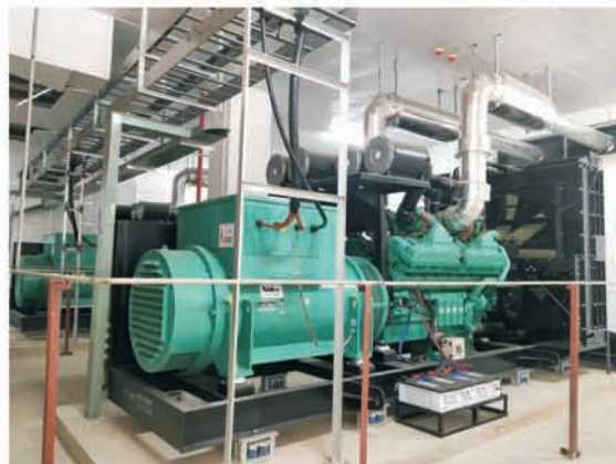
Project: Hunan Huayun Data Lake Units: 1800kW*2 Cummins City: China Hunan
