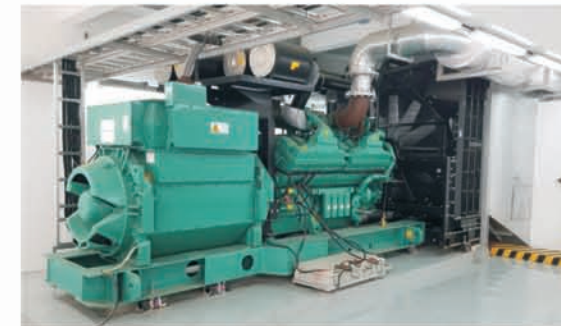
Project : Jiangsu HengYun Cloud Model & Units : 10.5KV R-C2500D5A * 6 City : China-Jiangsu
