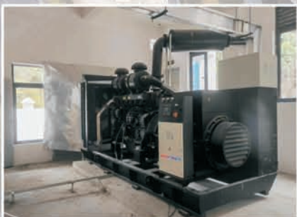
Project: Renzun Expressway Units: 700kW SDEC City: China Guizhou
