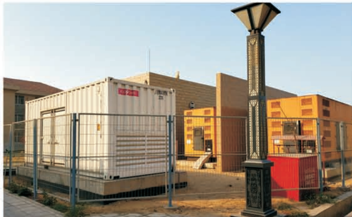
Project : Kasim Coal-fired Power Plant Project in Pakistan Model & Units : R-P1500S * 2 City : Pakistan
