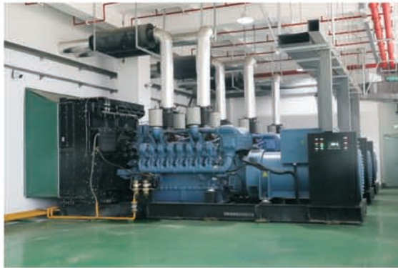
Project: Data Center Chinanet Wuxi Units: 1800kW*5 MTU City: China Jiangsu
